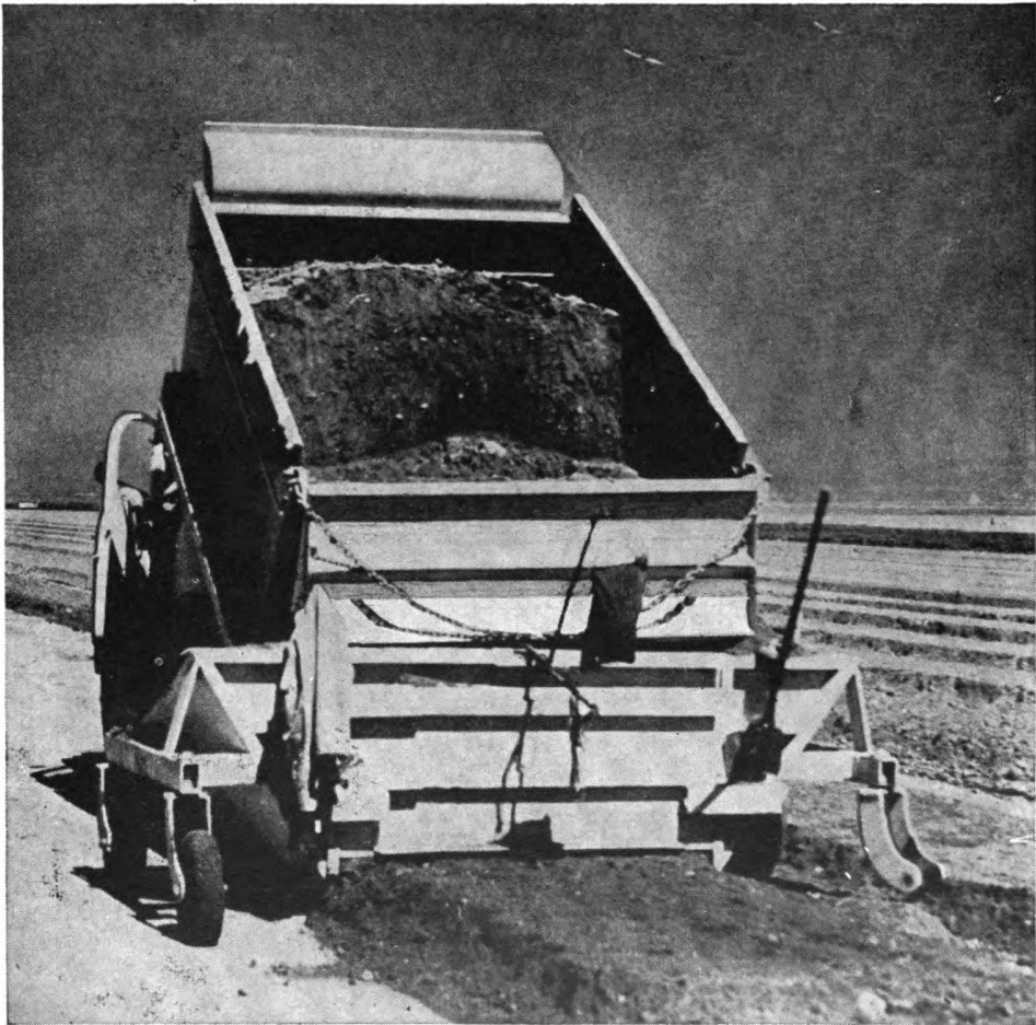
Figure 70. Processed base material being spread from truck onto runway subgrade, using spreader box.
